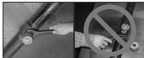
CORRECT (Piping is in place at the ceiling) INCORRECT (Sprinkler at floor level)
